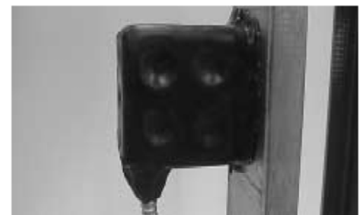
Step 6: Trim excess putty from corners and apply it to conduit fittings or cables connected to the box. Ensure pad is pressed firmly to surface of top, back, bottom, and side of box.
